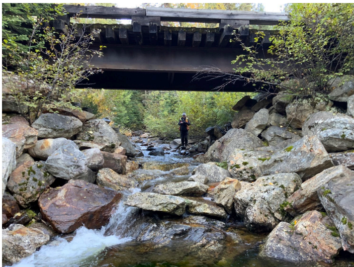
Photo 13. Looking northeast at an approximately 11 m long forestry road bridge approximately 3.9 m above Hummingbird Creek. The bridge is approximately 4 km upstream of the fan-delta apex.
