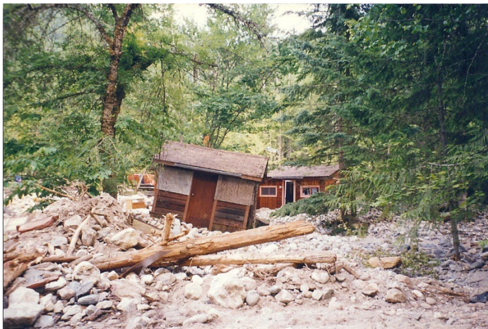
Photo 31. Looking at damages to unknown buildings on the upper fan-delta due to the Hummingbird Creek debris flow on July 11, 1997.
