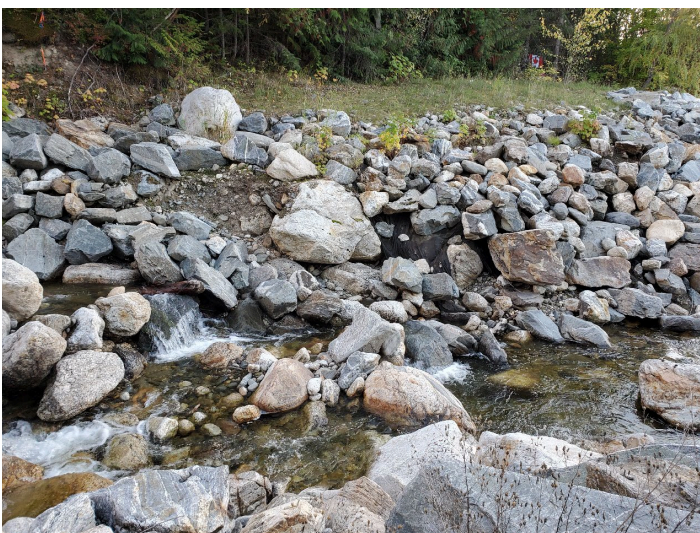
Photo 19. Looking south (across channel) at the condition of the rip rap along the south (left) bank of Hummingbird Creek upstream of the Highway 97A bridge. Note the black fabric (geotextile) visible next to the riprap.
