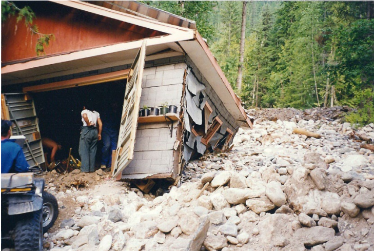
Photo 30. Looking at damages to an unknown building on the upper fan-delta due to the Hummingbird Creek debris flow on July 11, 1997.
