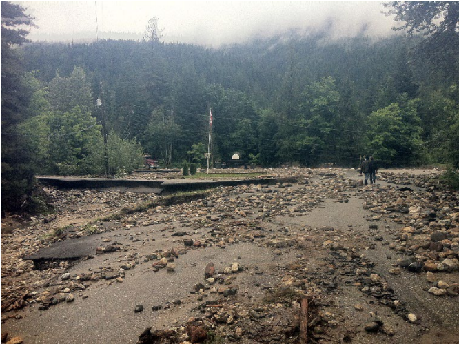
Photo 36. Looking east at Swansea Point Road, Highway 97A, and the Hummingbird Creek avulsion channel following the 2012 debris flood.
