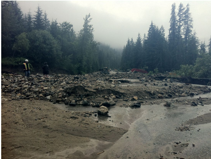
Photo 34. Looking south at the Highway 97A Hummingbird Creek culvert crossing following the 2012 debris flood.
